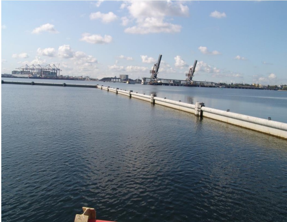
Permanent anti-spill barriers inside the terminal between jetties P and R
