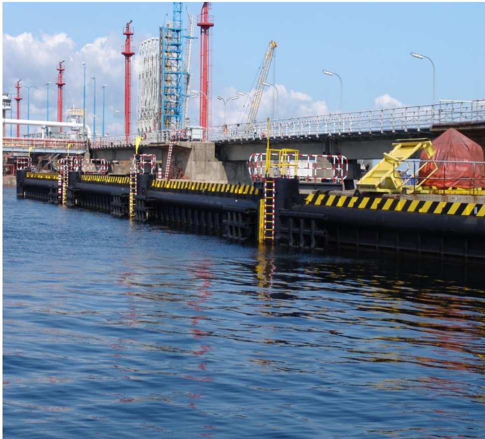
Anti-spill protection pneumatic barriers on a seabed which separates cargo handling basins
